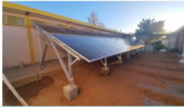
PV system installed at a school
